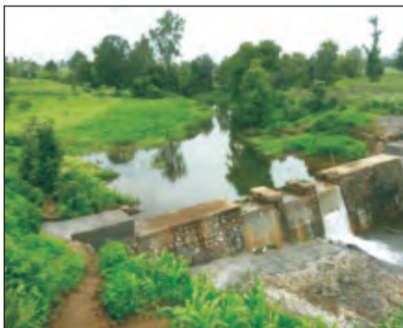
A water conservation scheme/percolation tank/check dams in Nirugudi village of Satara district
